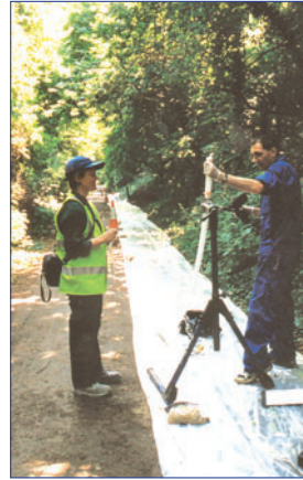
CMT System installed to a 60 m (200 ft) depth with seven monitoring zones. Installation was completed by placing layers of sand and bentonite to monitor a BTEX/MTBE plume in a Chalk aquifer, United Kingdom.
