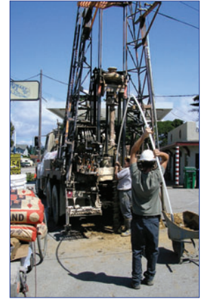
A gas station site in Watsonville, California. Five 3-Channel CMT Systems were installed to monitor gasoline contamination and MTBE plume. Installations were completed within hollow stem augers using bentonite and sand layers to isolate each monitoring zone.
