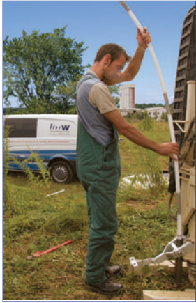
3-Channel CMT installation at a plant in Zeitz, Germany. Systems were completed using natural collapse and are being used to assess natural attenuation of BTEX.
